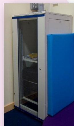
1 x Control Cupboard
