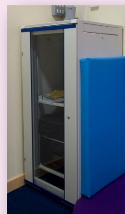
1 x Control Cupboard
